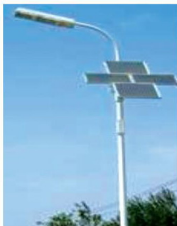
Solar Street Light
